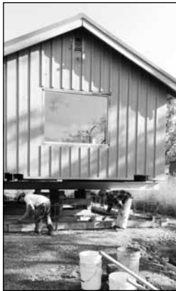
Workers added finishing touches as the Baker House foundation was poured in perfect weather on October 25.
