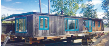
This house from the “Sleepless in Seattle” floating neighborhood now rests happily on Orcas.
