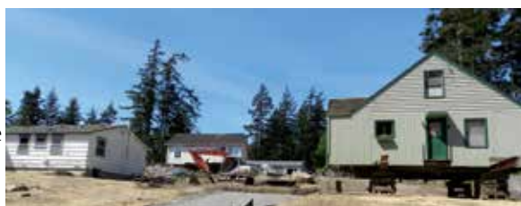
Three recently moved houses that are being renovated by OPAL on Seaview Street.
